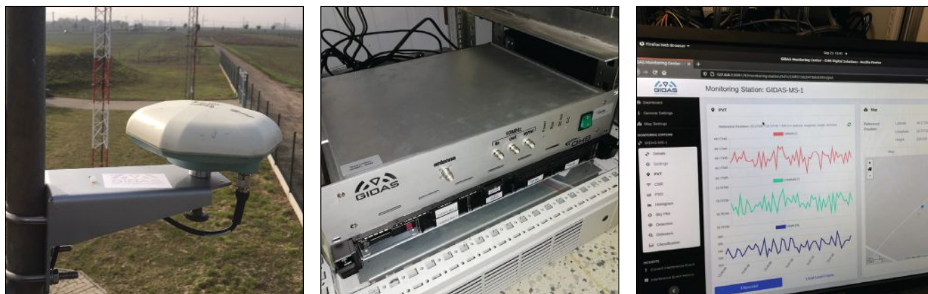
FIGURE 7 Installation of monitoring station (left: antenna mounting on mast; middle: RFFE and SDR in server rack; right: monitoring system user interface).
